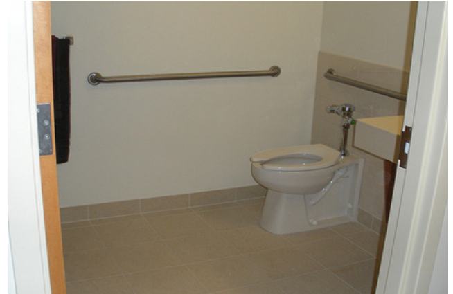
Bathroom installation of WarmlyYours TempZone™ electric radiant floor heating
